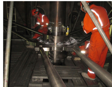
Chemical—Steady bearing inspection
