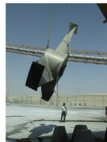
Mining—SX Impeller retrofit
